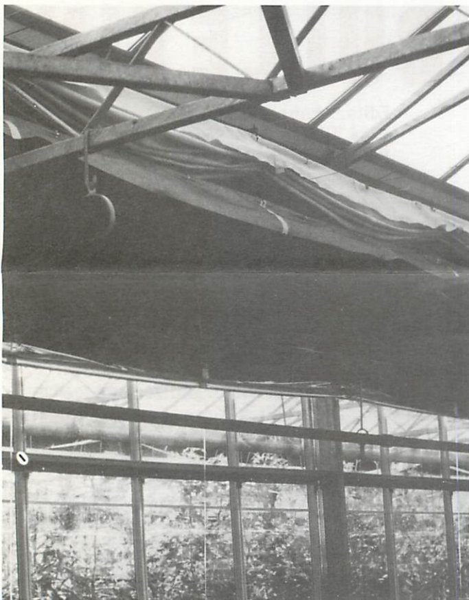
Figure 2: Thermal screen, shade and black-out systems were installed in many glasshouses.
