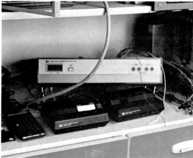
Fig. 3. Installation of the system for control in a remote, air-conditioned room. For any system of this type, protected location, and security of the controls is important. This requires suitable cabling and connections which costs might equal or exceed the acquisition expense of the basic system.
