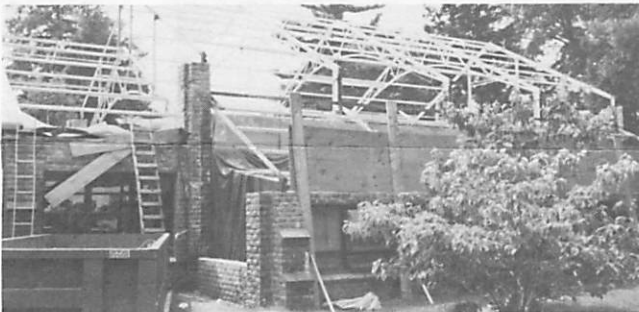
Plywood was used to build a platform over the plants so work could be done on the high trusses.
