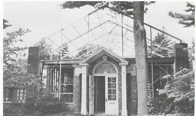
The Camellia House at Planting Fields during the reconstruction of its framework.
