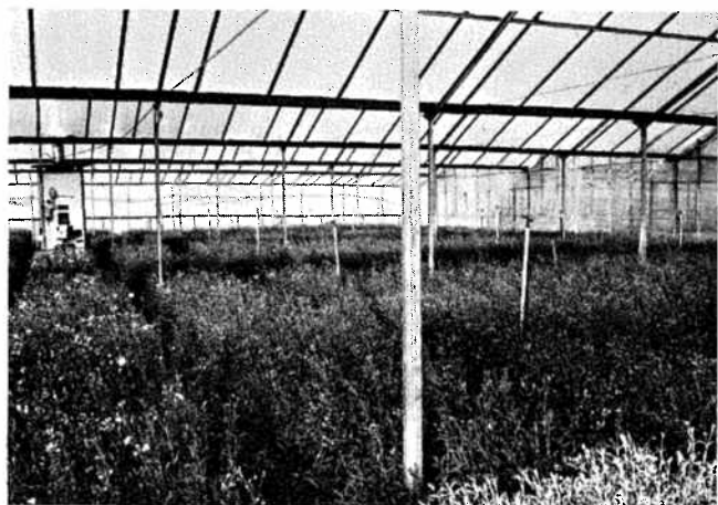
Fig. 1: Typical heater installation in a polyethylene-covered range of miniature carnations. Carnation ranges are seldom heated and this one is the exception. Rose ranges use similar heaters.
