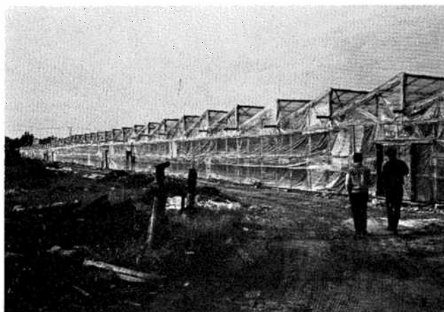
Fig. 2: Some "Southern California" plastic construction for roses in Israel.
