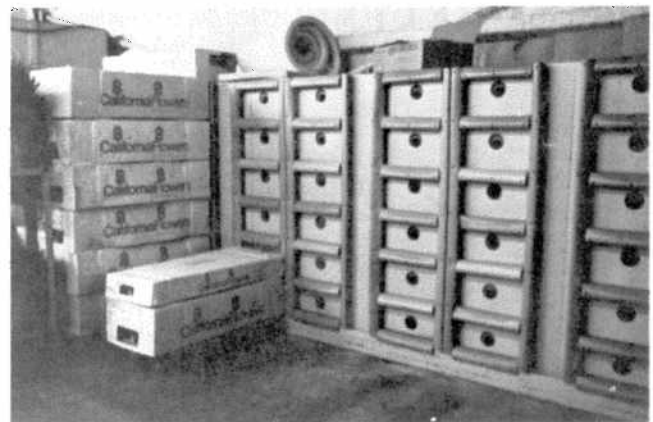
Figure 4: Typical forced-air cooling system to be found in several locations. The flower box is pushed against the sections with air being forced through the packed box.
