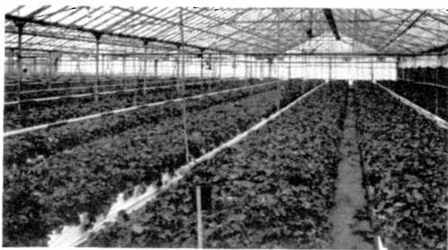
Figure 6: Yoder Brothers' propagation range in the Watsonville region. Note the infra-red radiant heating tube along the ridge of this Geranium house. Installation recently completed with significant savings in fuel costs compared to the conventional piped steam.
